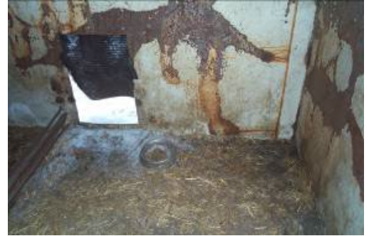
8-21. No bedding, rusted dog enclosure 3.1(c)(1)(i); 3.3(a)
