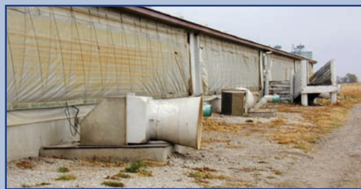
Manure Pit Fans and Side Curtains
