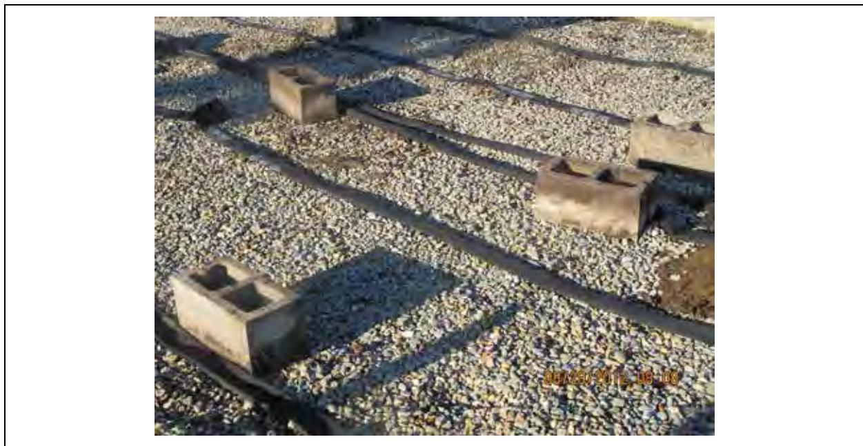
Figure 14-2 Concrete Blocks Used to support Tarp from Surface to Allow Steam Distribution from Steam Sock
