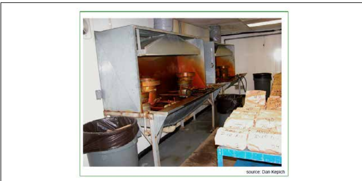
Figure 4-5 Fenwick Can Washers in Sample Washroom
