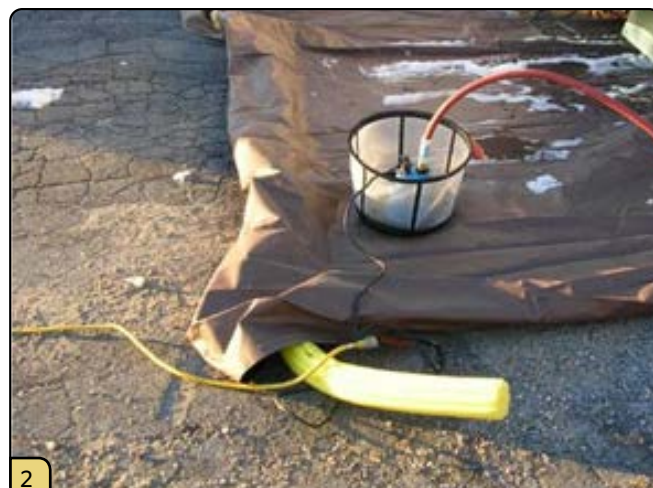
2 Sump pump in bucket strainer.
