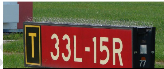
Figure 1. Porcupine wire installed at an airport to prevent perching birds (e.g., raptors).
