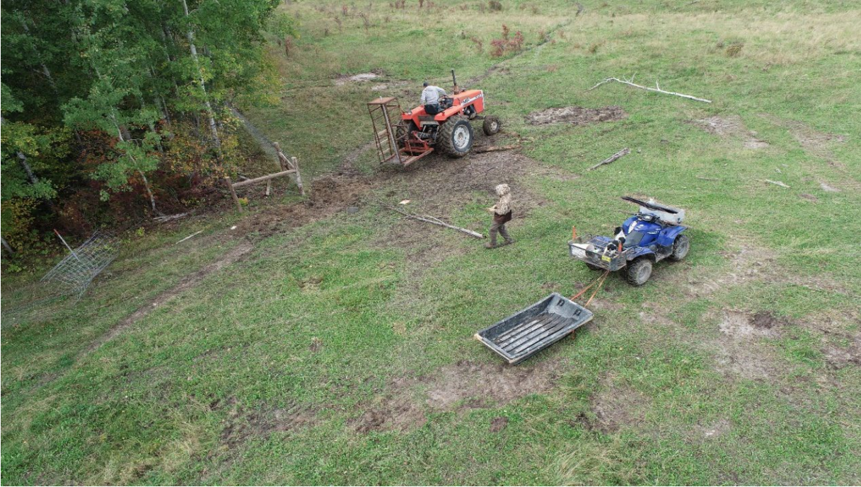
Figure 2. WS Staff Working with Producer to Install Permanent Fence. (Sheep Ranch, St. Louis County)
