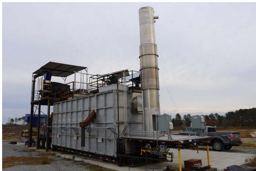
Figure 3. Opposing Side View of Gasifier
