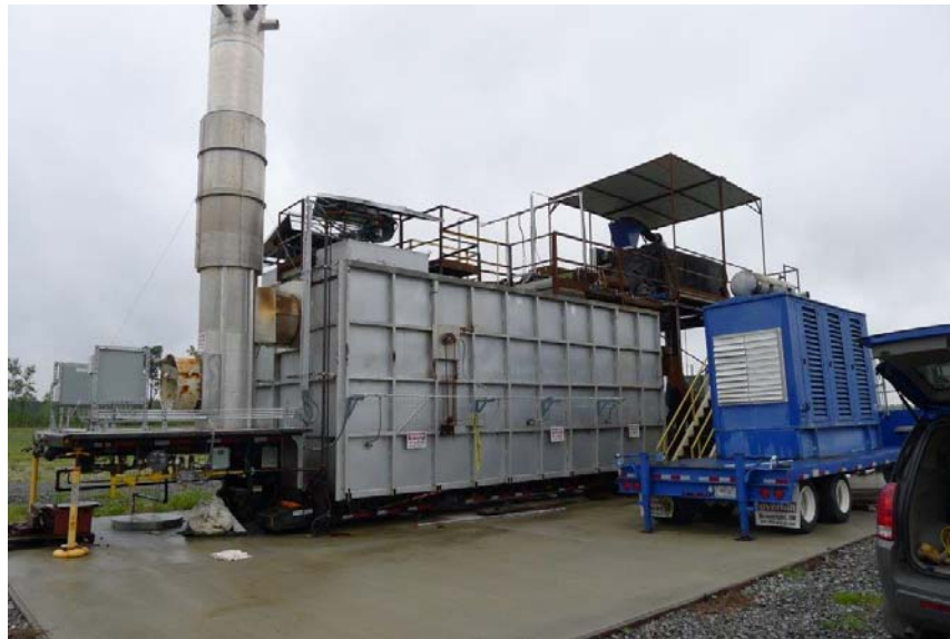
Figure 2. Front View of Gasifier and Diesel Generator
