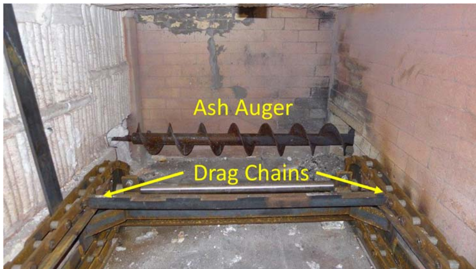
Figure 8. Gasifier Chamber Showing Drag Chains and Ash Auger
