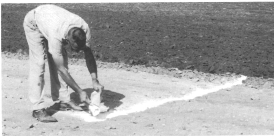
FIGURE 40.—A 6-inch band of lime is placed on the surface of soil to check efficiency of plowing operation. N-38175
