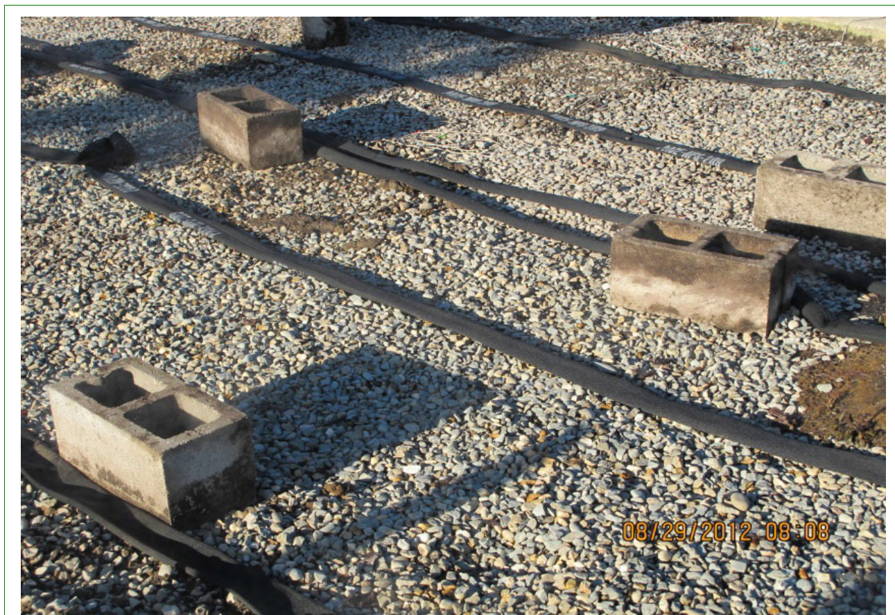
Figure 12-1-2 Concrete Blocks Used to Support Tarp from Surface to Allow Steam Distribution from Steam Sock
