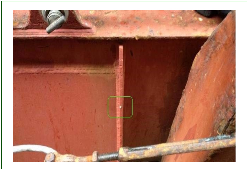
Figure 2. FSMC Eggs Found Between Two Bays on a Support Beam Near a Cargo Hold Opening (Figure 2 illustrates FSMC eggs found between two bays on a support beam near a cargo hold opening.)
